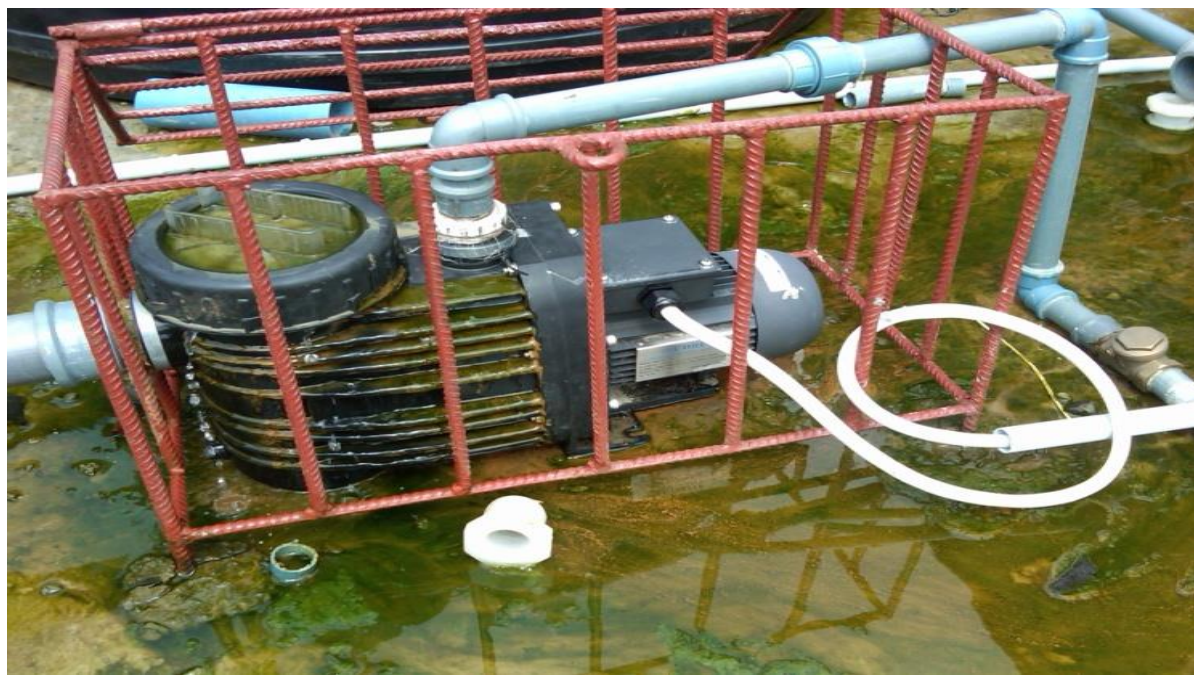
Leaking surface water pump of the solar PV installation at Ide Village
