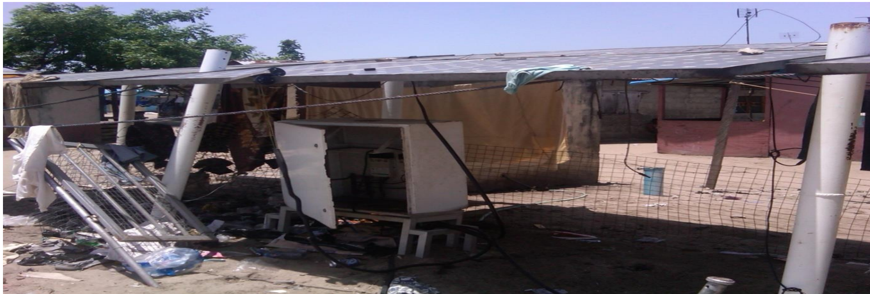
The non-functional Solar PV Installation Sagbokoji Village
